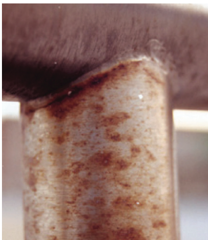
Severe tea staining of stainless steel in a coastal environment shortly after installation.
