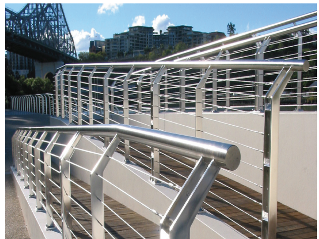
Holman Street, Brisbane: Example of successful use of stainless steel in a marine environment.
